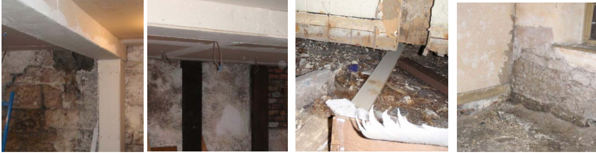
Downstand beam & Column Additional timbers at Wall Unsupported Partition Exposed solum
