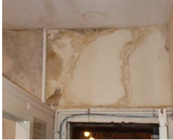
Damp at common gable
