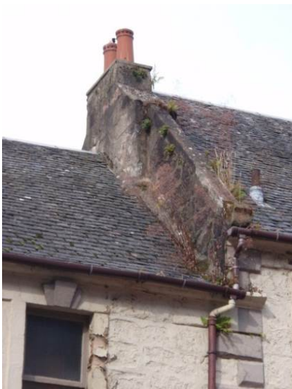
Weed growth, blocked gutters and open joints in stonework
