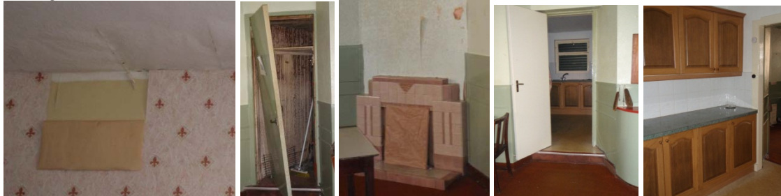
Peeling Wallpaper, some mould growth
